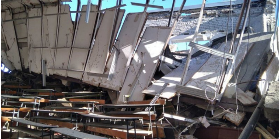
Picture 1: The academic building of the Karazin University Institute of Physics and Technology was significantly destroyed.
