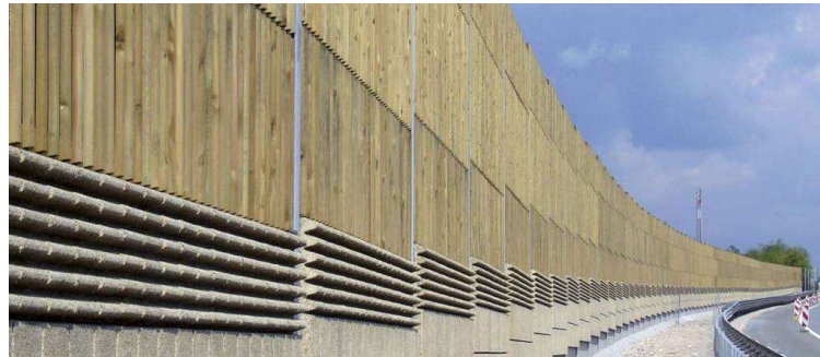
Fig. 6.13 Wooden noise reduction barrier
