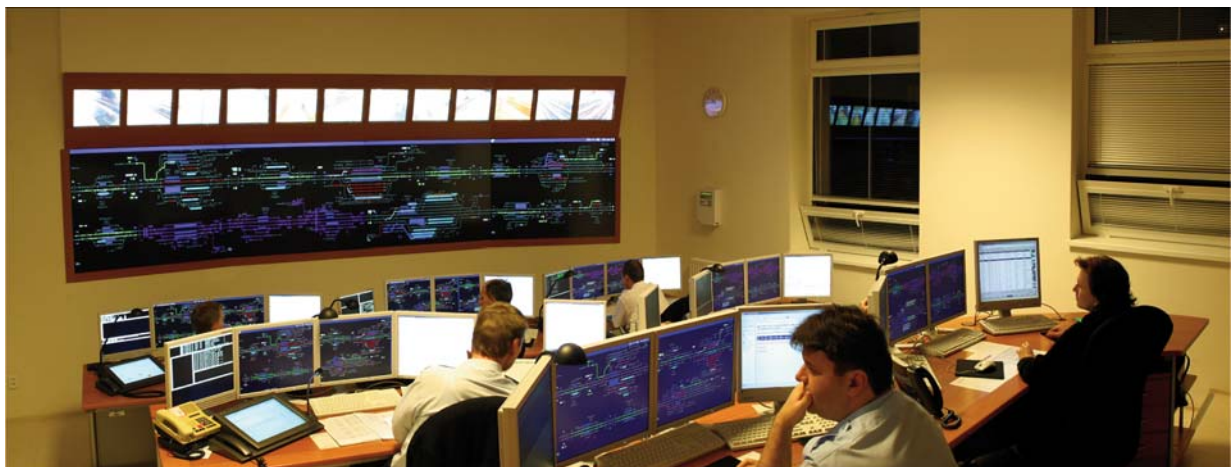
Fig. 1 CDP Prerov, Large dispatcher's room No. 1 – General view of the dispatcher and operator centralised control place
