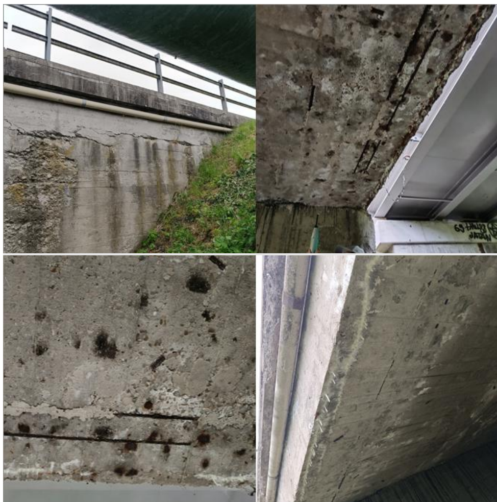
Figure 3 Defects on bridge M7441 (Figuli 2025)
