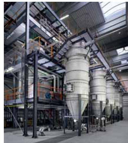
Instalace u BOR-BIOTECHNOLOGY
