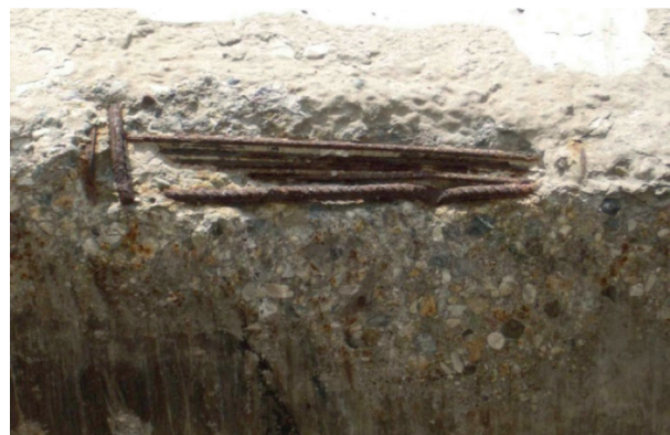
Fig. 5 The partial rupture of wires of the prestressing tendon - bridge No. 065-086
