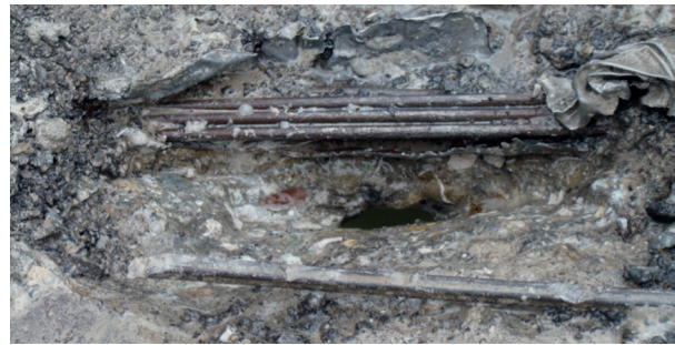
Fig. 4 The partial rupture of wires of the prestressing tendon - bridge No. 059-091
