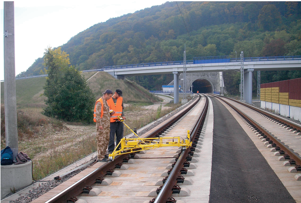
Fig. 3 View of the slab track structure in the area of earthwork (diagnostics of the alignment of track of the track using the KRAB™-Light device)
