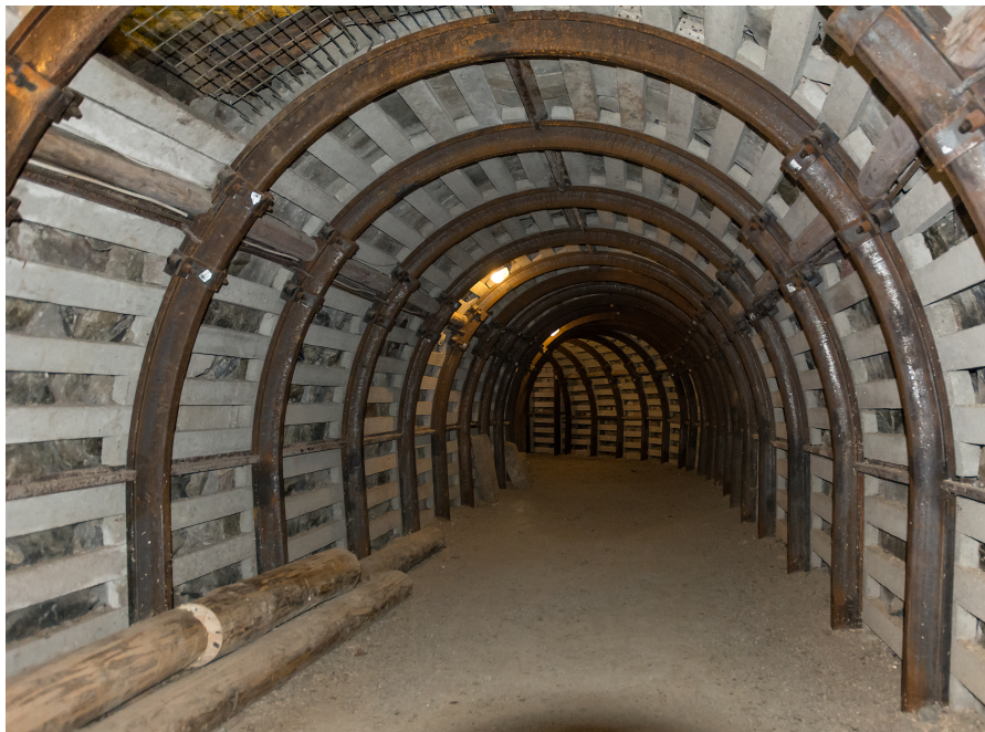
Fig. 5: View of steel arch yielding support ( https://upload.wikimedia.org )
